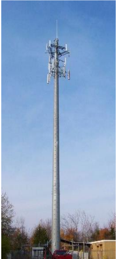
Macro Tower (4G) (monopole)
