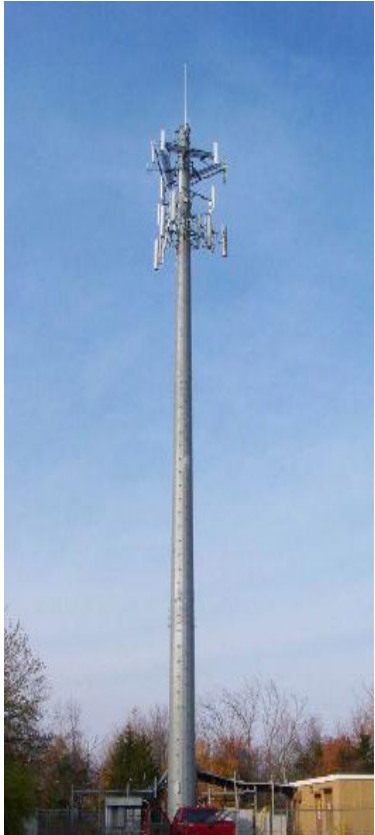
Macro Tower (4G) (monopole)
